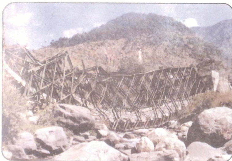
Photo 17 Collapsed Gawana gad bridge in Uttarkashi Maneri road sector.
