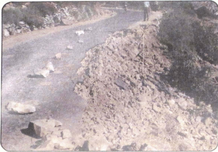
Photo 6 Failure of the valley side portion of block top road near Mannpur.
