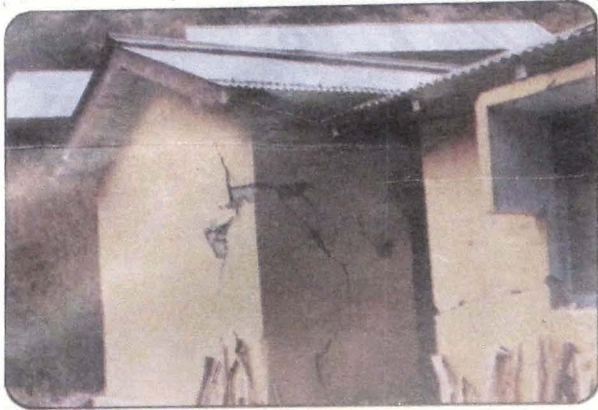
Photo 106 Cracks in walls of the staff quarters of Okhimath Public Health Centre.
