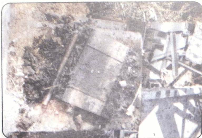
Photo 19 A Clockwise rotation of the downstream end baseplate, Maneri side of Gawana bridge. Rollers and roller plate not seen as they have been thrown in the river below.
