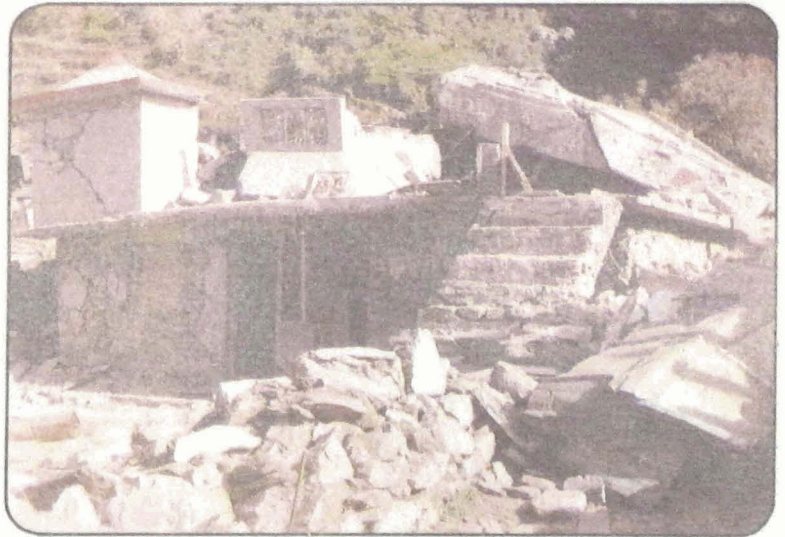
Photo 70 Collapse of first floor of a house in Byala Tipri village with deep open cracks in the ground and first floor. (New construction).
