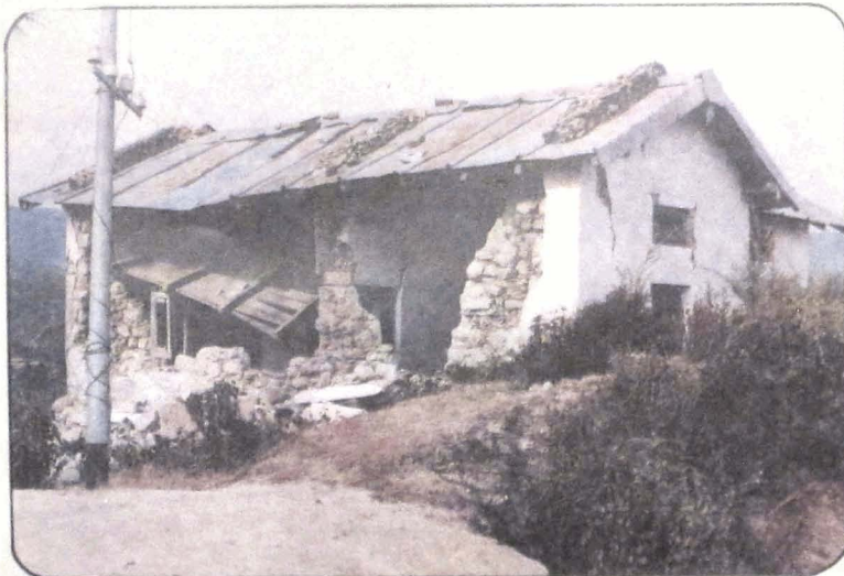
Photo 86 Collapsed veterinary hospital in Jakholi village.
