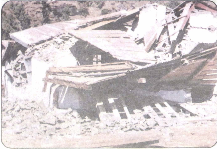
Photo 35 Complete collapse of forest rest house at Aghora.
