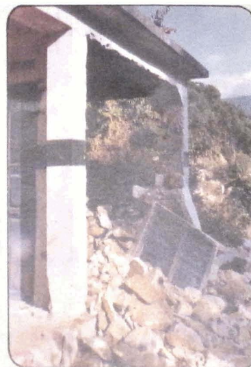
Photo 42 Complete collapse of a non-load-bearing masonry wall of Heena School.
