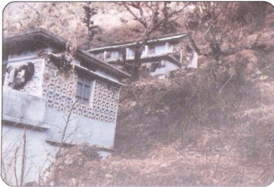
Photo 110 Plaster fall of the house in foreground and partial short wall collapse of the house in the background at Gaurikund.
