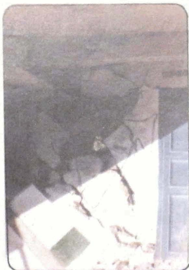
Photo 43 Prominent shear cracks in the side wall of Heena school.
