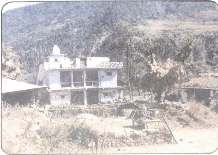
Photo 32 Shear cracks in the ground and first floors of a house in Ghorsali village.
