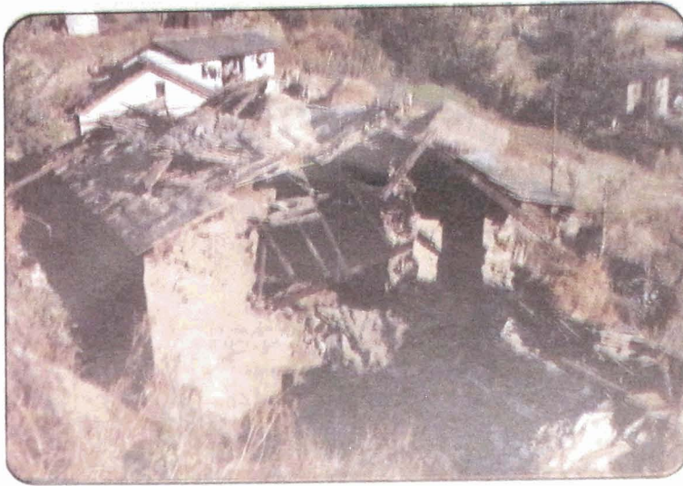
Photo 49 Partial to total collapse of thick mud masonry walls in Kamar village.
