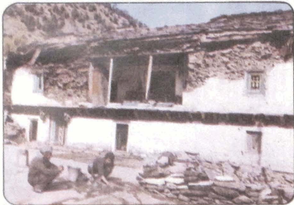
Photo 108 Partial collapse of first floor long wall of a house in Trijugi Narayan.
