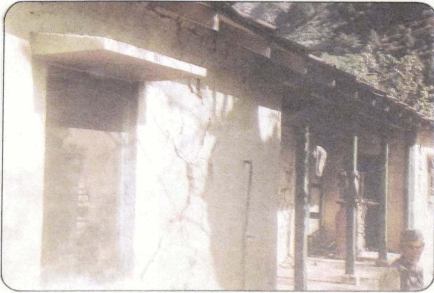
Photo 77 Open shear cracks in the out house of PWD rest house at Lambgaon.
