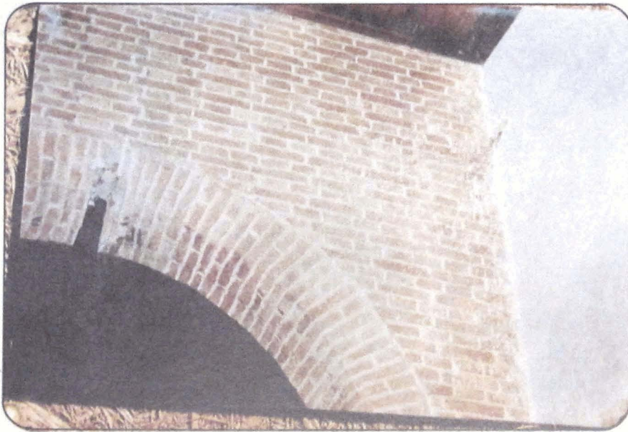
Photo 97 Dislodged brick from the centre of the arch portion of the first floor corridor-FRI building Dehradun.
