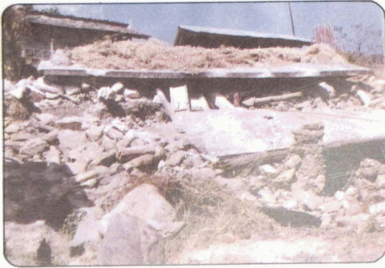
Photo 66 Collapse of houses with RCC slabs in Mannpur village. Note relatively lesser damage to the conventional houses in the background.
