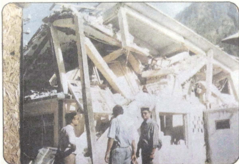
Photo 24 Collapse of the first floor of RCC, State Bank of India building in Uttarkashi.
