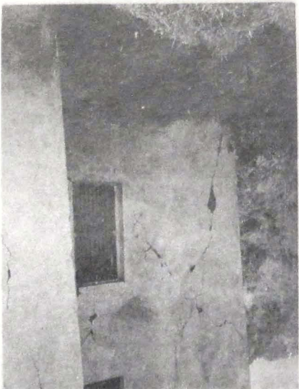
Photo 104 Collapsed house in Timbi village.
