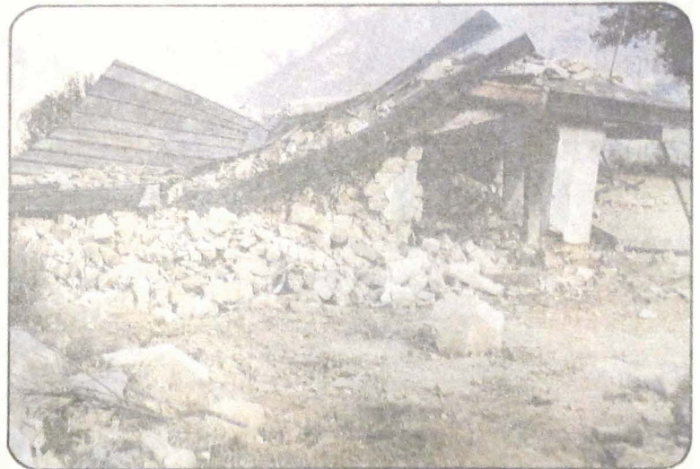
Photo 33 Complete collapse of a school building in Jakhol village.
