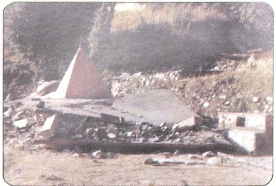
Photo 48 Collapse of a temple in Jamak village. Note intact pyramidal portion of the temple and damaged RCC roof slab.
