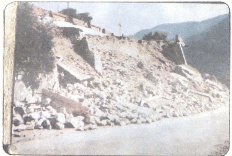
Photo 2 Failure of buttressed breast wall of the approach road to Maneri colony. (Photo NGRI).
