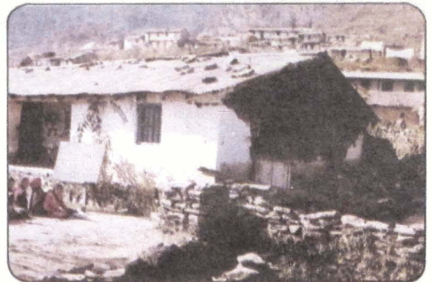
Photo 109 Collapse of short wall of the School building, Trijugi Narayan.
