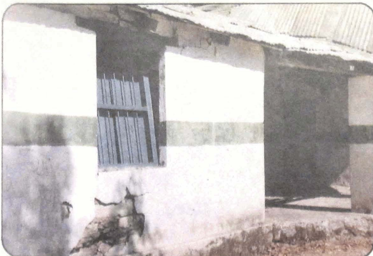
Photo 34 Tilted window of a school at Aghora and partial collapse of partition walls.
