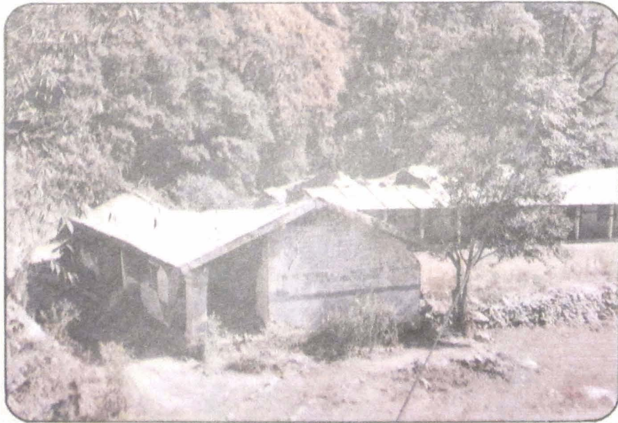
Photo 36 Collapse of the northern wall of a school building at Kalyani.
