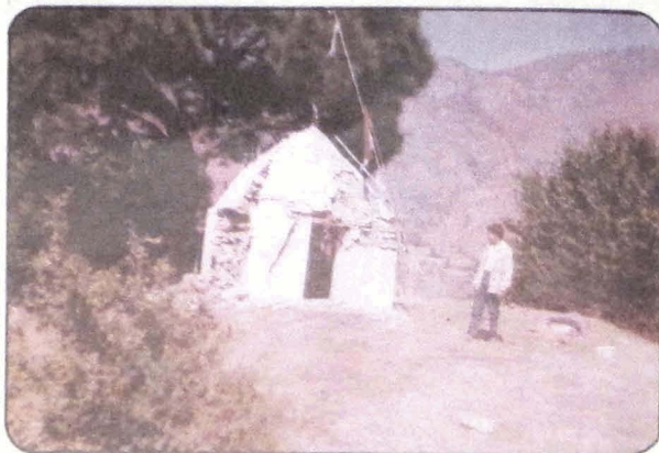
Photo 92 A Damaged lowrise roadside temple, a few km before Barkot along Kalsi-Barkot road.
