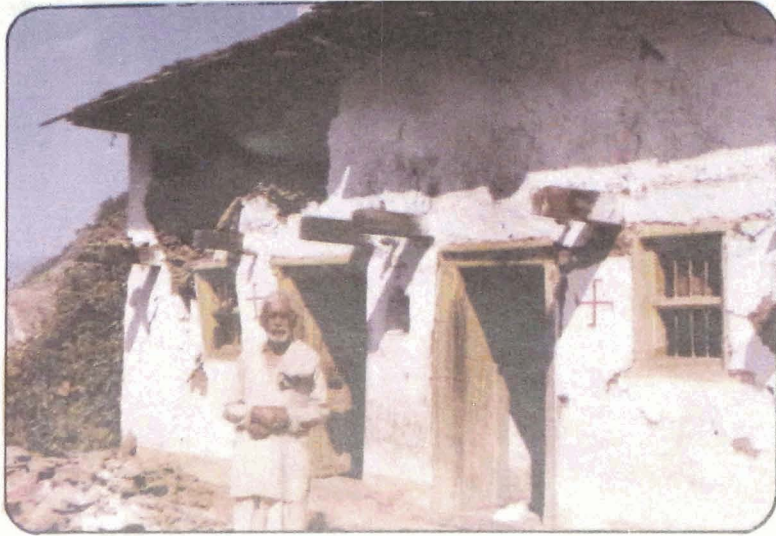
Photo 69 Partial collapse of the roof corner of the first floor of a house in Thalán village.
