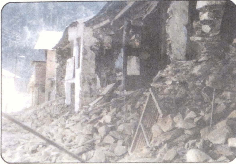
Photo 20 A view of collapsed house of Shri Ram Lal, adjacent to the Nagar palika building is Uttarkashi town.
