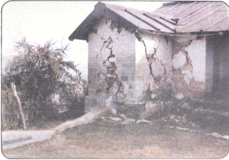
Photo 84 Damaged residence of doctor in Jakheli village.
