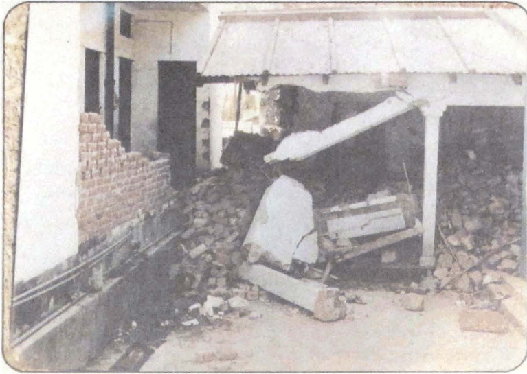
Photo 22 Collapse of pillar and beam of the verandah of a house in Police Lines, Uttarkashi.
