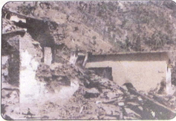
Photo 37 Collapse of a kutch house of Ganeshpur village. The adjoining brick masonry house has suffered much less damage.
