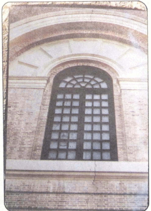
Photo 96 Cracks in the arch and sill portion, in the rear wall of FRI building.
