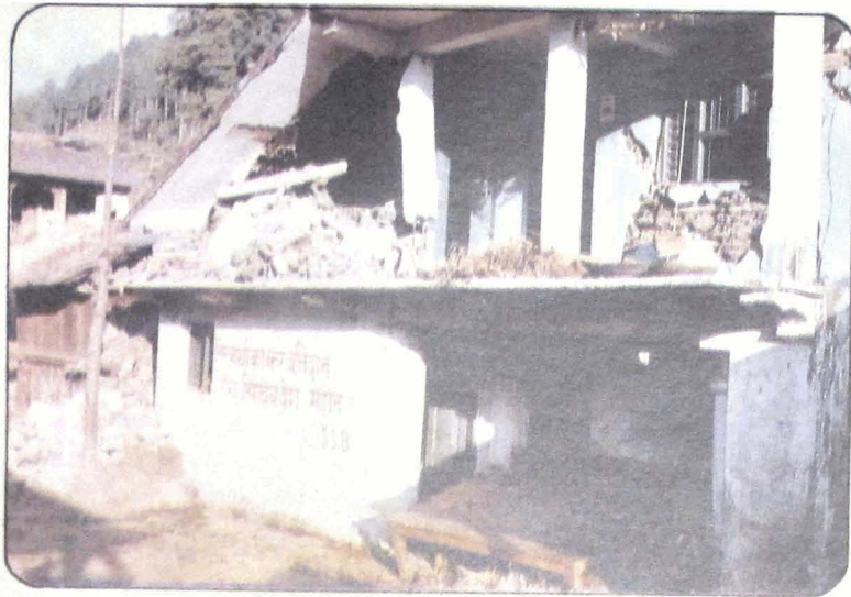
Photo 52 Partial collapse of the first floor of a house in Dedsari. Note damages to RCC pillars and open shear cracks.
