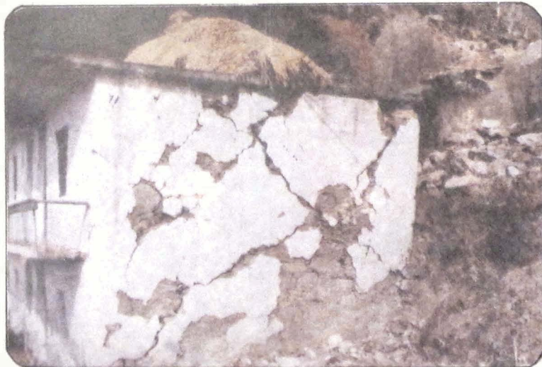
Photo 83 Heavily sheared side walls of a house in Gorthi village.
