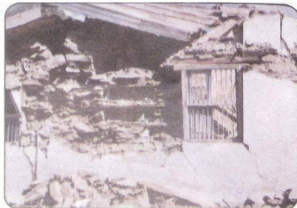
Photo 57 Partial collapse of mud masonry side walls of school building in Raithal village.
