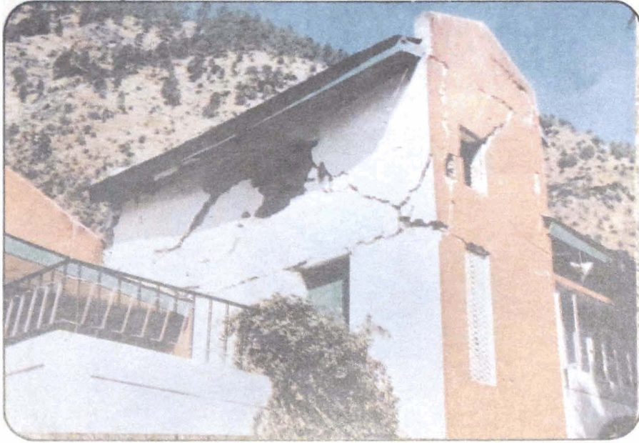
Photo 27 Heavily damaged first floor of the Maneri Inspection house with shear cracks in both long and short walls.
