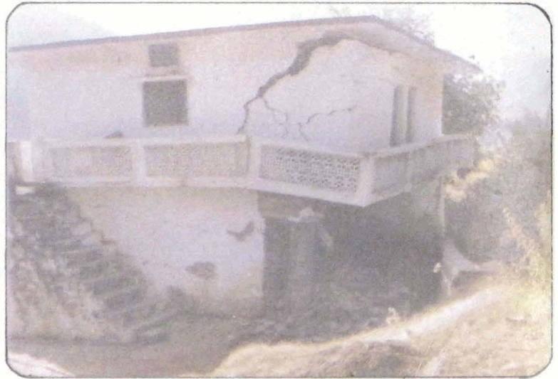
Photo 73 Tilting of the first floor frontage of a double storey house because of the collapse of the ground floor wall in village Gyansu.
