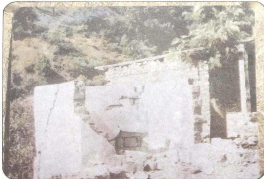
Photo 26 Damages in a low height structure in Gangeri village. (Photo NGRI).
