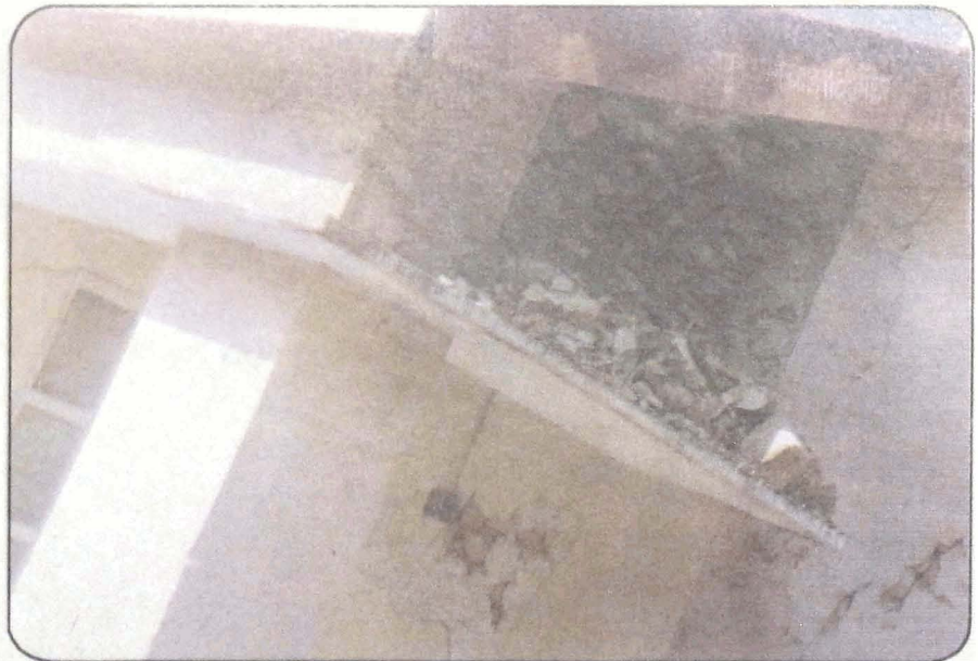
Photo 78 Damage to side walls of the PWD rest house at Lambgaon.
