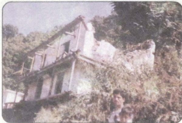
Photo 89 Collapse of first floor of a conventional house in Gangani village.
