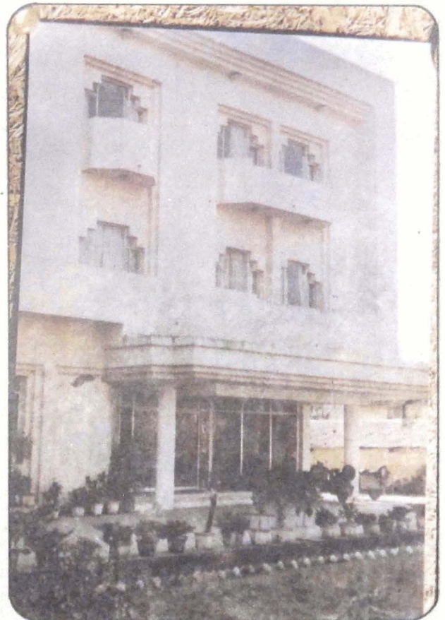
Photo 98 Fall of plaster and development of cracks in the panel wall adjacent to the porch-Hilton Hotel, Dehradun.
