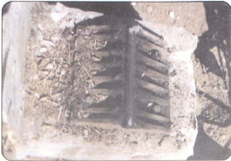
Photo 18 Intact base plate of the rocker on the Uttarkashi side of the Gawana bridge.
