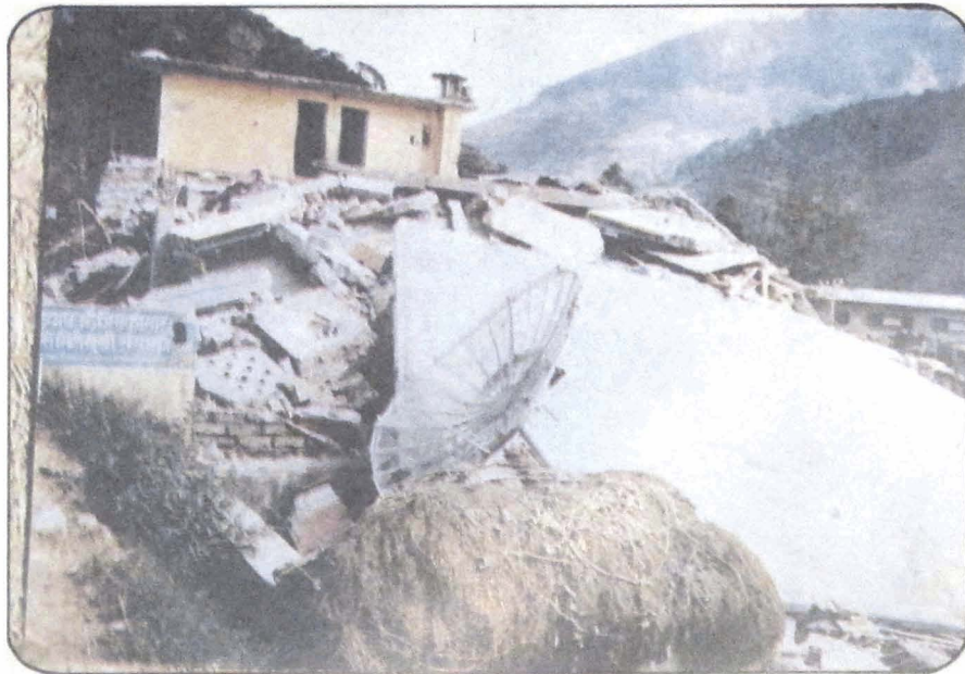
Photo 30 Complete collapse of a house with RCC roof at Aungi village. Note relatively much less damage in a house at the top left corner.
