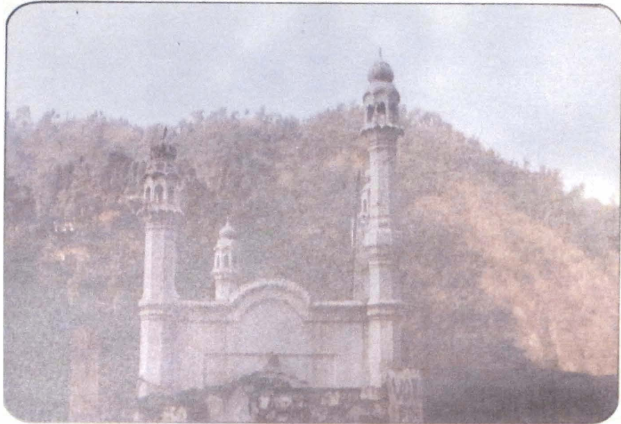
Photo 114 Horizontally cracked minaret of a mosque, Dugadda.
