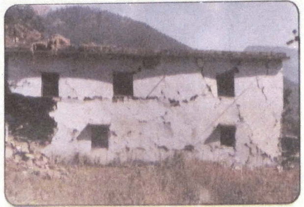
Photo 38 Collapse and cracks in the long walls of a house in Ganeshpur village.
