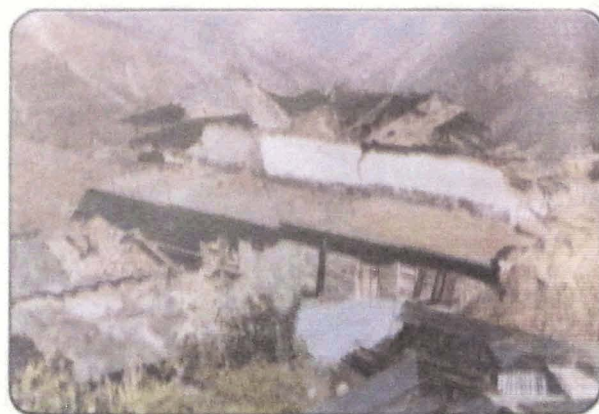
Photo 58 Extensive damage to conventional type-A houses. Collapse of walls and resultant breaking of concrete slab in one of the houses in Raithal village.
