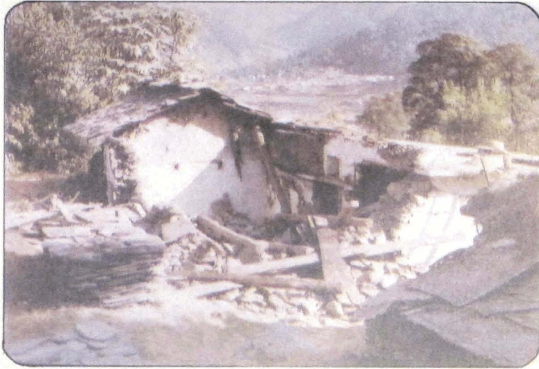
Photo 72 Collapse of cluster of houses in Gyansu village.
