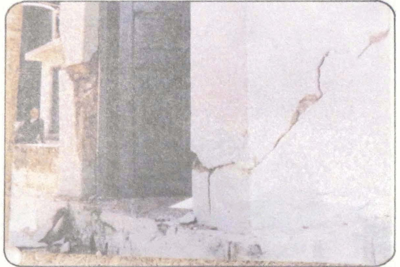
Photo 28 B Shear cracks in one of the houses in Maneri colony. (Photo NGRI).
