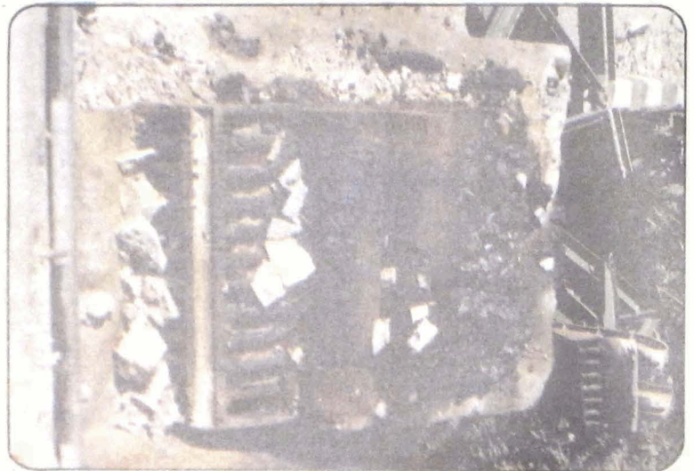
Photo 19 Upstream end intact base plate on the Maneri end of the Gawana bridge. Note rollers in place and slipped roller plate and coupling rod in the foreground.
