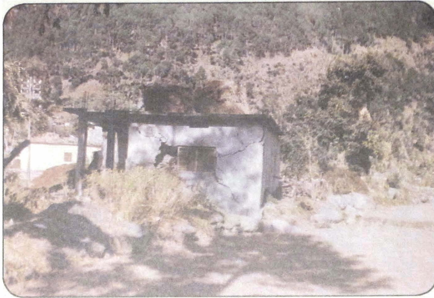
Photo 25 Shear cracks in the E-W aligned side wall of a house in Gangeri village.
