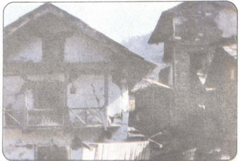
Photo 64 View of an old conventional house with wooden beams and columns displaying gaping shear cracks in Siror village.
