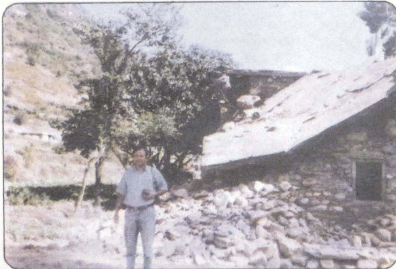
Photo 74 Failure of the stone masonry wall leading to sagging and partial collapse of a RCC roof slab in Matti village.
