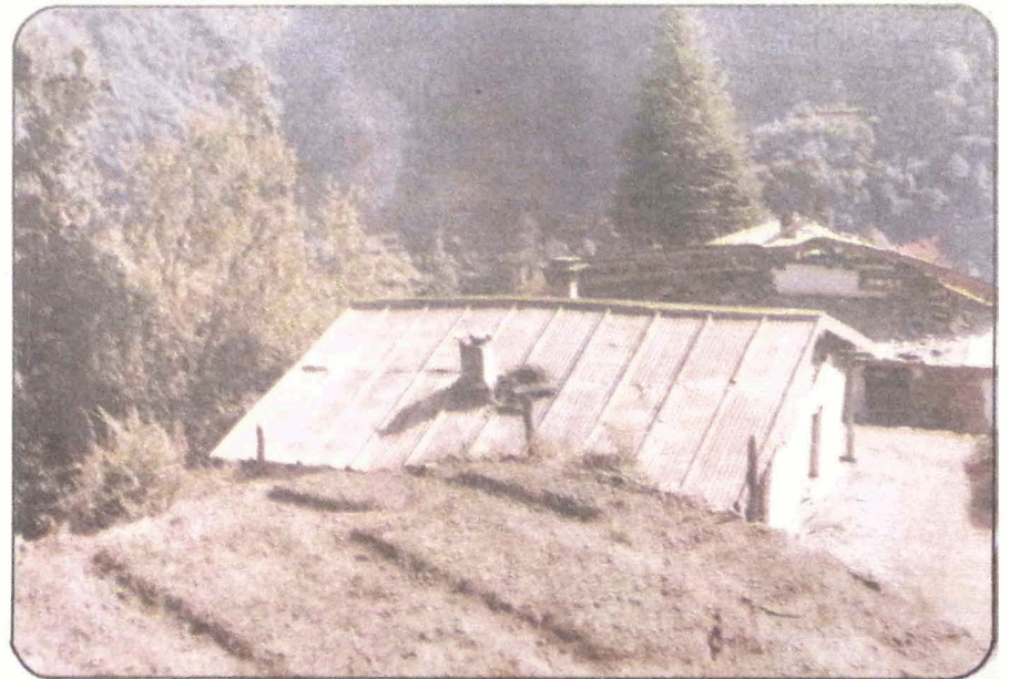
Photo 60 Damaged PWD Rest house building, Bhatwari. Chimney slab of the out house thrown on G. I. sheet roofing.
