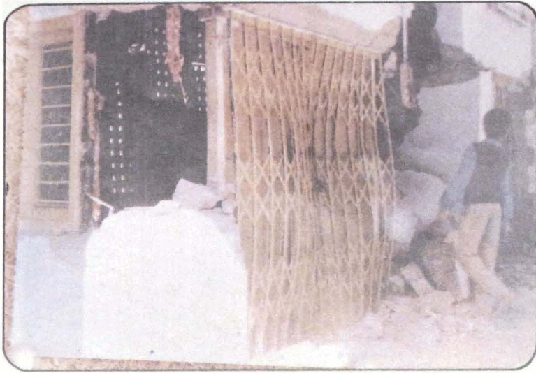
Photo 28 A Collapsed walls and buckled shutters of the temple in Maneri project colony. (Photo NGRI).
