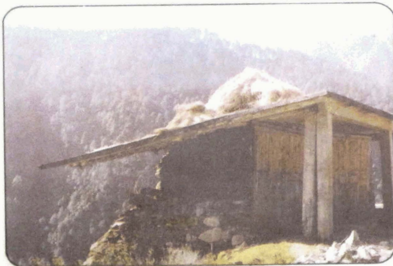
Photo 68 Sagging and collapse of RCC slab supported on mud masonry walls in a house in Thalan village.
