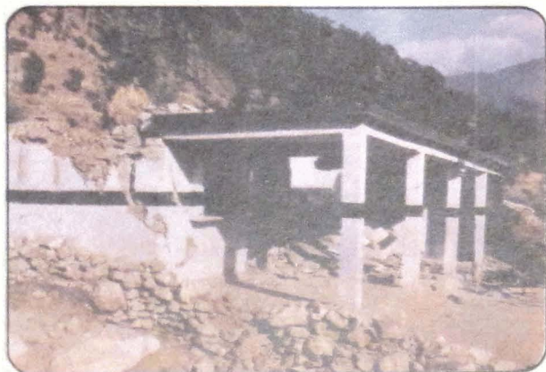
Photo 41 Severely damaged school building in Heena.
