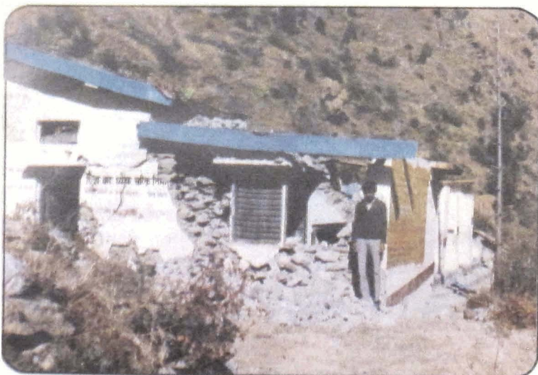
Photo 55 Collapsed school building in Sanglai village.
