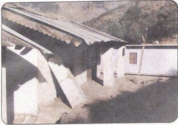
Photo 87 Tilting and collapse of pillars of a house in Rana village.
