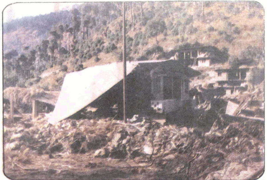
Photo 46 Damaged houses in Jamak villages. Note severed and tilted RCC roof slab.
