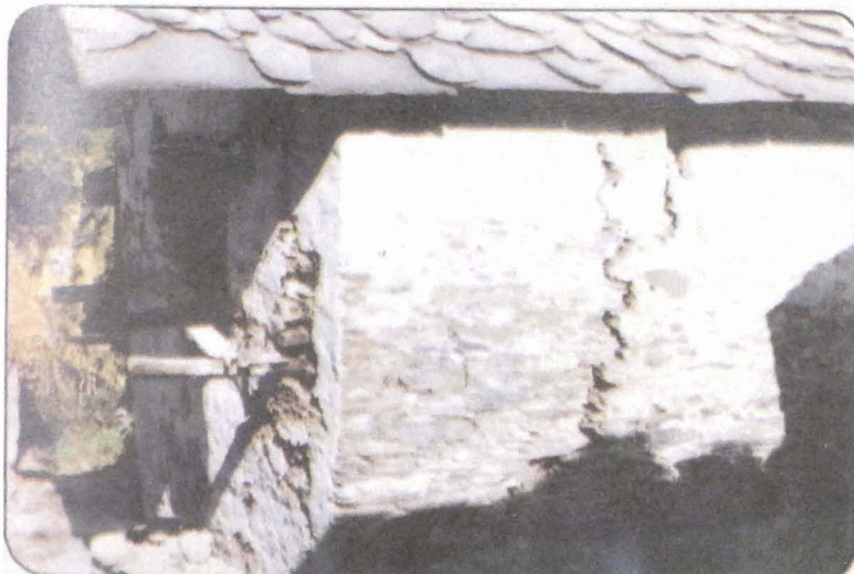
Photo 65 Bulging and cracking of thick masonry walls of a house in Siror village.
