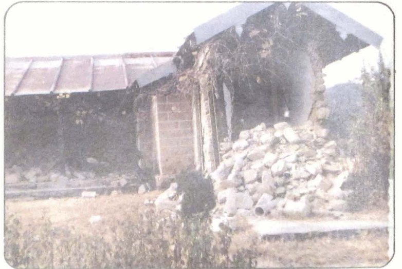
Photo 85 Collapse of a type-B house in Jakholi village located on a spur.
