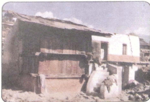
Photo 94 Bulging and cracking of walls of a house in Purola village.
