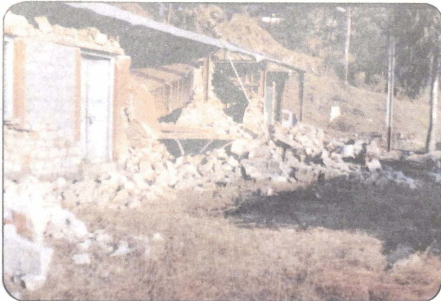
Photo 28 Collapse of single storey office complex in Maneri dam colony.
