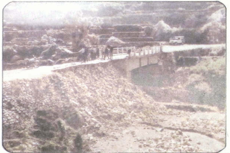
Photo 7 Damaged approaches of the bridge over river Indravati near Kishenpur. See undamaged RCC bridge of about 15 m. span.
