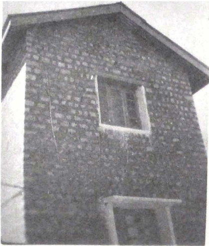
Photo 102 Bulging of the west wall of double storey Rest house at Chitkul.
