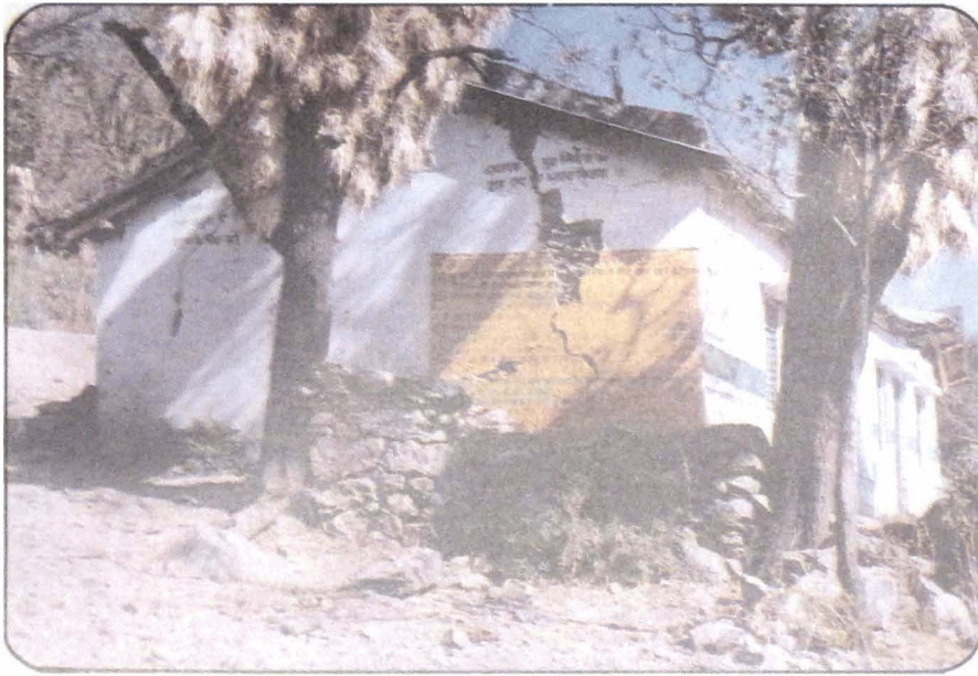
Photo 61 Shear cracks in the side wall of Pala school building made in mud masonry.
